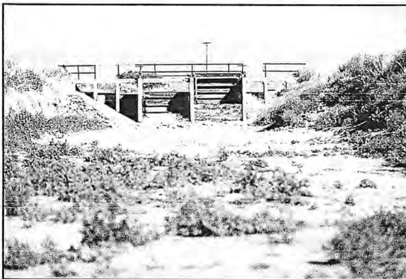
Dry Canal, Klamath Irrigation Project. Photo courtesy of Klamath Water Users Association.
